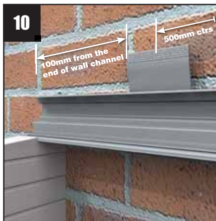
10 Offer the wallplate up to the wall and position it so that the top surface of the bolt slot is level with the top of the firrings.
