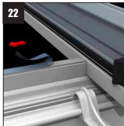
22 Tease the 'tail' of the glazing support trim tape free (ready to be pulled away when the sealed unit is finally in position).
